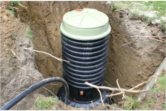
1). Grinder pump (Initial Installation)
